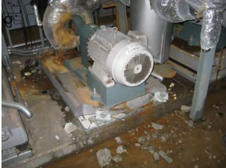
Fig. 2 Damage at the base of a pump
