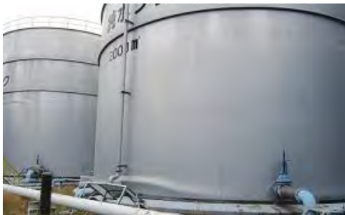
Fig. 10 Buckling failure of a 2,000 m 3 water tank (Thermal and Nuclear Power Engineering Society, 2011)
