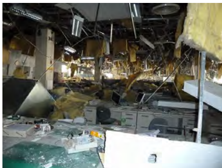
Fig. 14 Fallen ceiling materials
