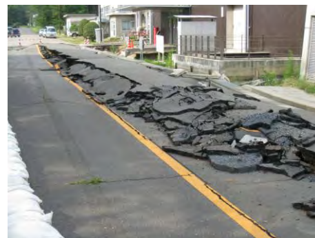
Fig. 19 Damage to road due to ground subsidence
