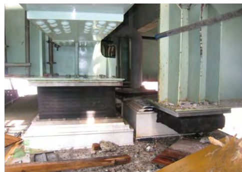
Figure 5 Damage to a bridge support
