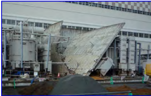
(c) Damaged concrete wall.
