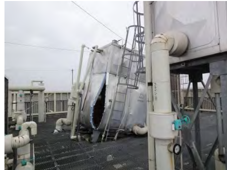
Fig. 5 Failure of a water tank installed on a roof
