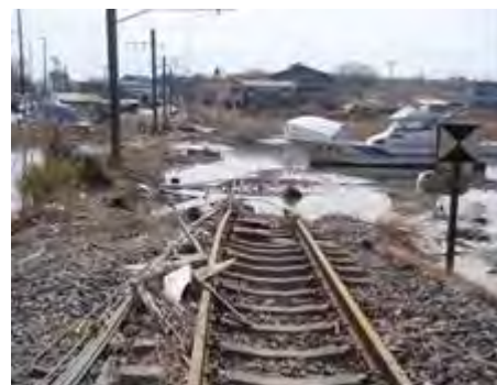
Fig.3 Washed away of track
