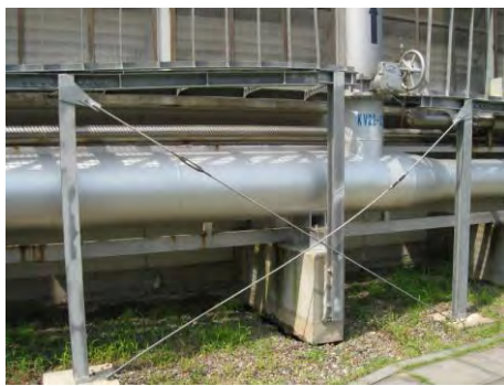
Fig. 16 Uplift of a pipe support base due to ground subsidence
