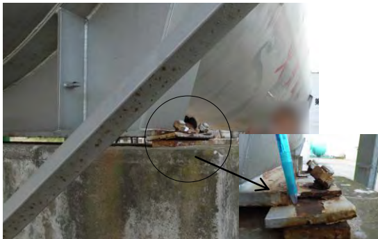
Fig. 20 Lifting damage to LPG tank by tsunami
