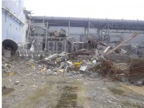
Fig.11 Debris that was scattered due to the hydrogen explosions
