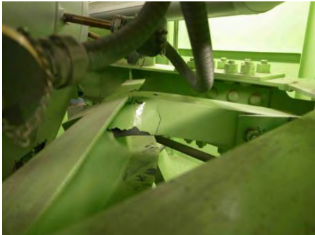
Fig. 6 Damage to the anti-vibration bar of a boiler
