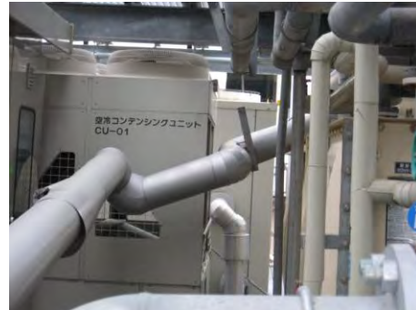
Fig. 7 Failure of a pipe support (in-house hanging pipe)
