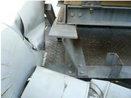
Fig. 4 Deformation of the steel base of a FRP tank
