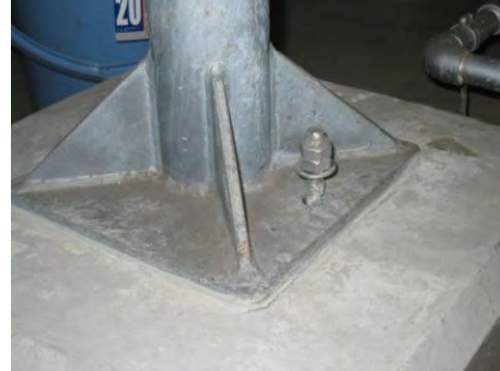
Fig. 3 Deformation of an anchor bolt (Provided by JAXA)
