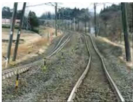
Fig.2 Subsidence of embankment
