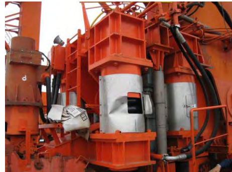
Fig. 24 Damage due to collisions with floating objects (Provided by TEPCO)
