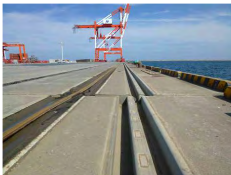
Fig. 18 Quay wall deformation and misalignment of the unloader rail
