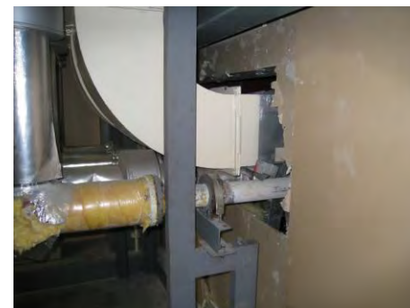
Fig. 9 Damage to inner walls by pipes (Provided by JAXA)
