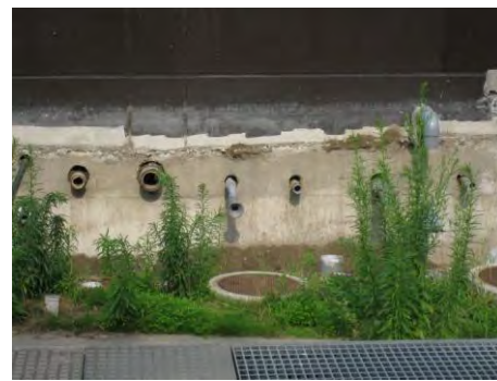
Fig. 17 Pipes fractured at the connection point of the building and soil
