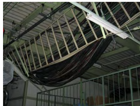
Fig. 15 Failure of cable racks
