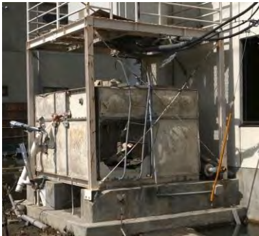
Fig. 23 Failure of a FRP tank caused by the tsunami
